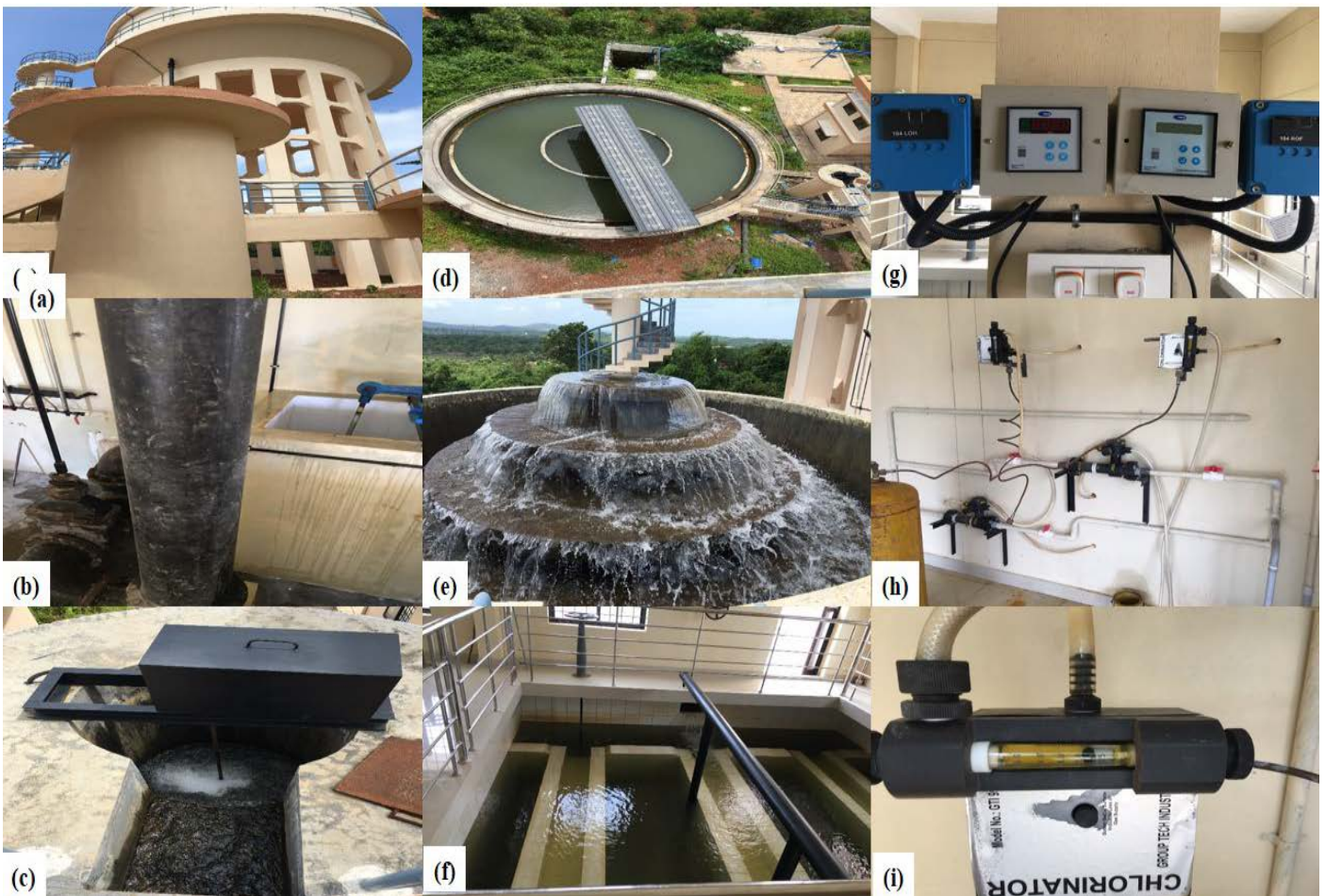
Figure 17: Photographic view of different components of water treatment plant (a) Overhead tank (b) Pipeline for water supply (c) Flocculent mixing chamber (d) Flocculation chamber (e) Aeration chamber (f) settling chamber (g) metering point (h) chlorination cylinder (i) chlorinator meter
