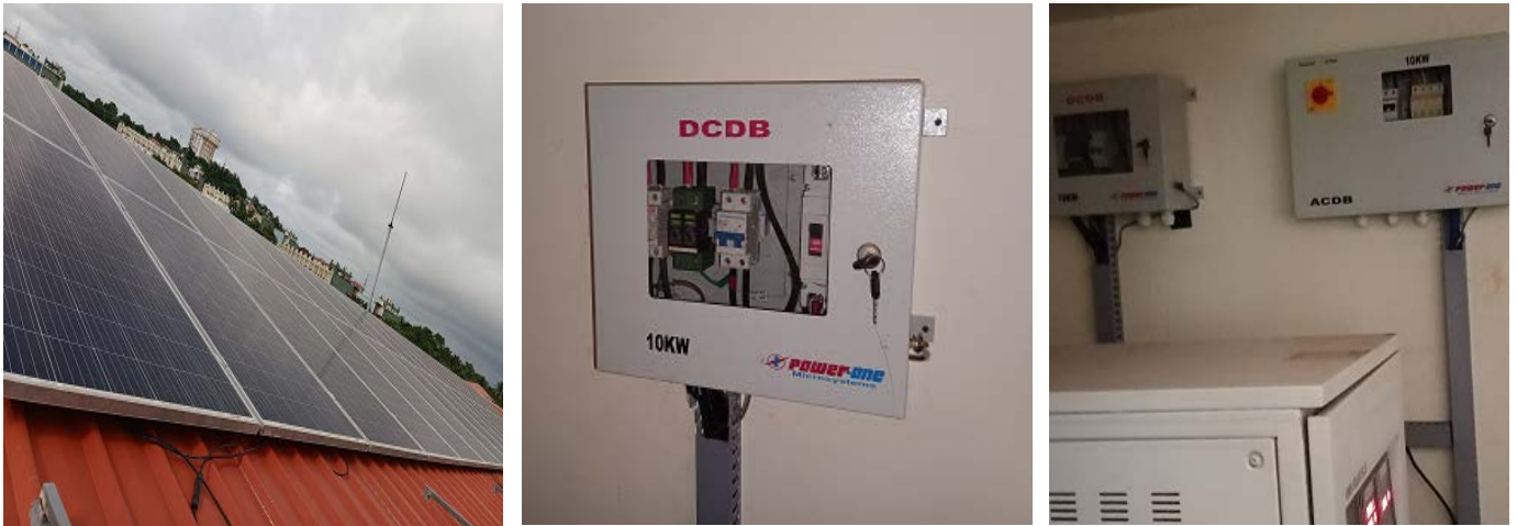
Figure 12: 10 KW Roof top solar panel
