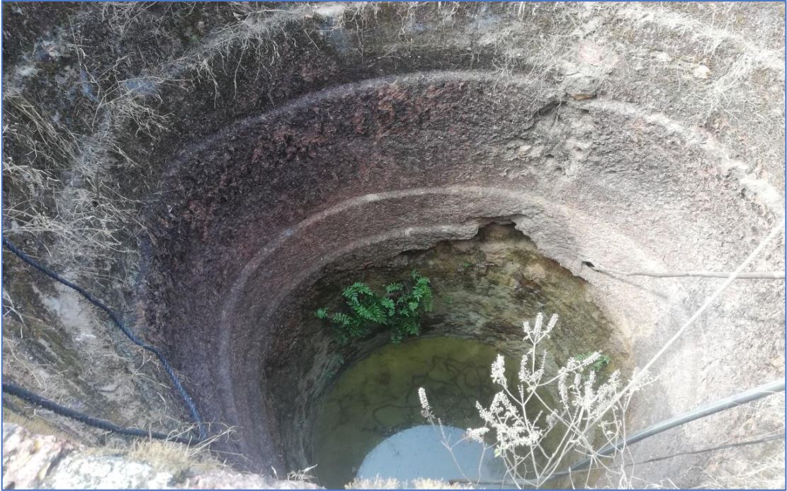
Fig. 4.3. Well No. 1 showing cracks and moderate turbulent water.
