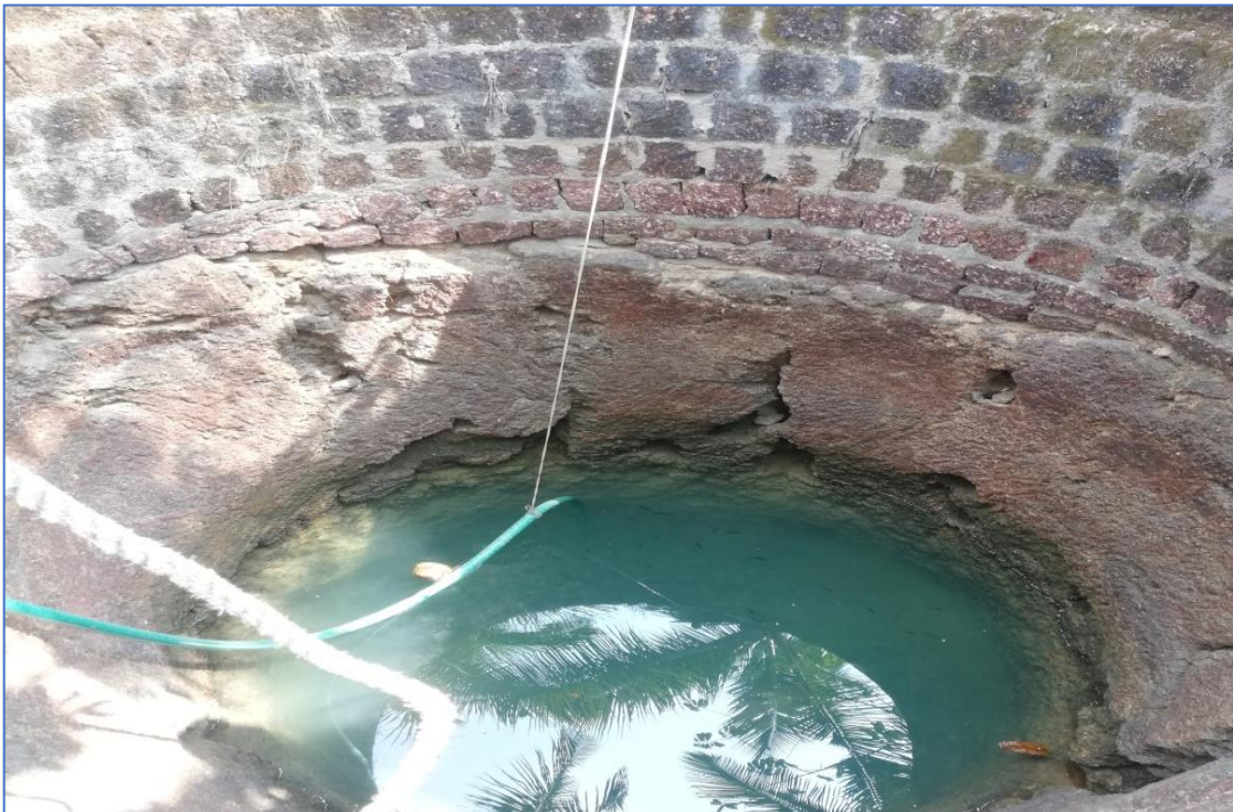
Fig. 4.4. Well No. 5 with cracks and clear water.
